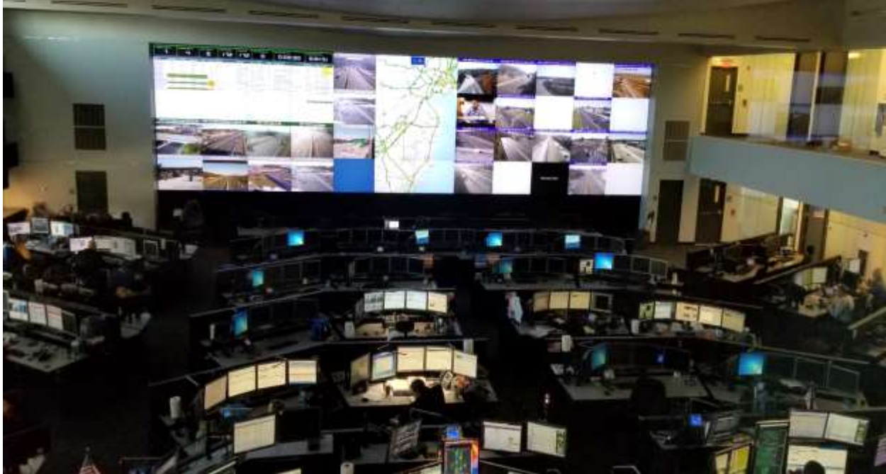
Figure 7. Statewide Traffic Management Center
